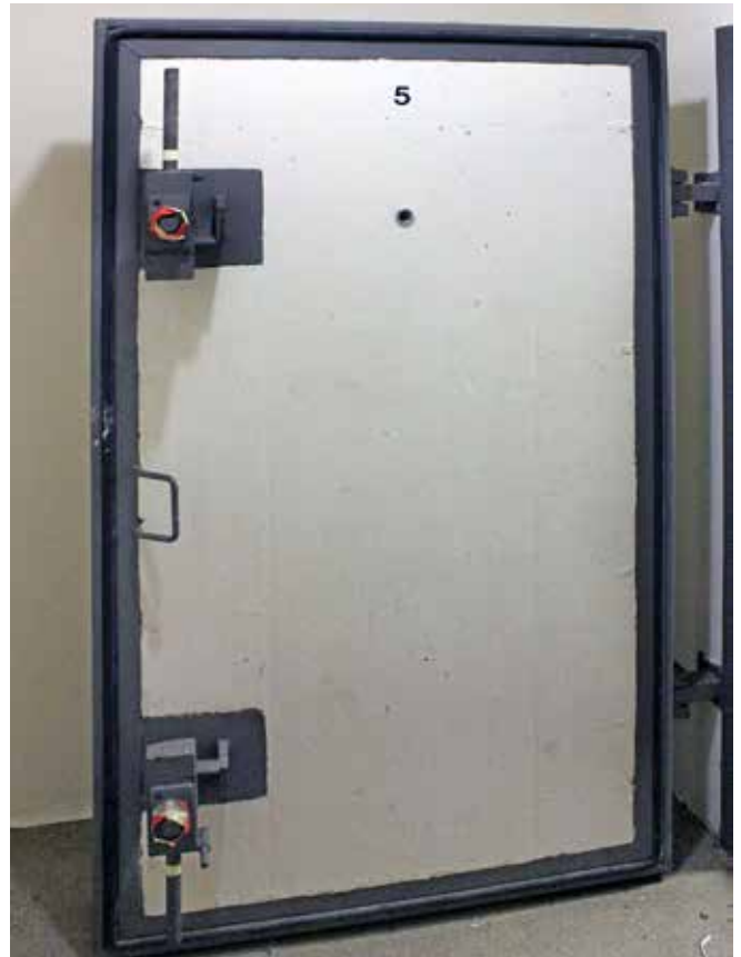
Reinforced concrete blast door leading to decontamination showers located on the upper level
